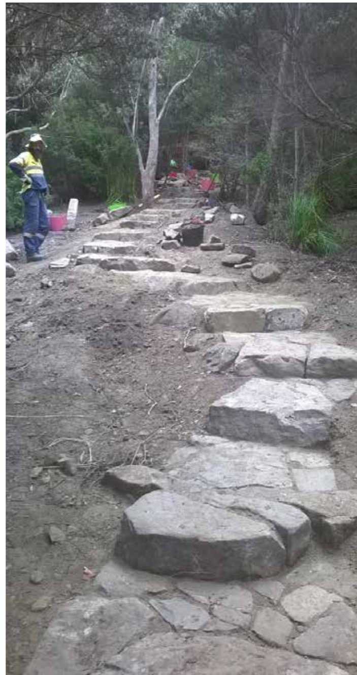
Photo: New stone steps at Radford's track Old Hotel loop road crossing
