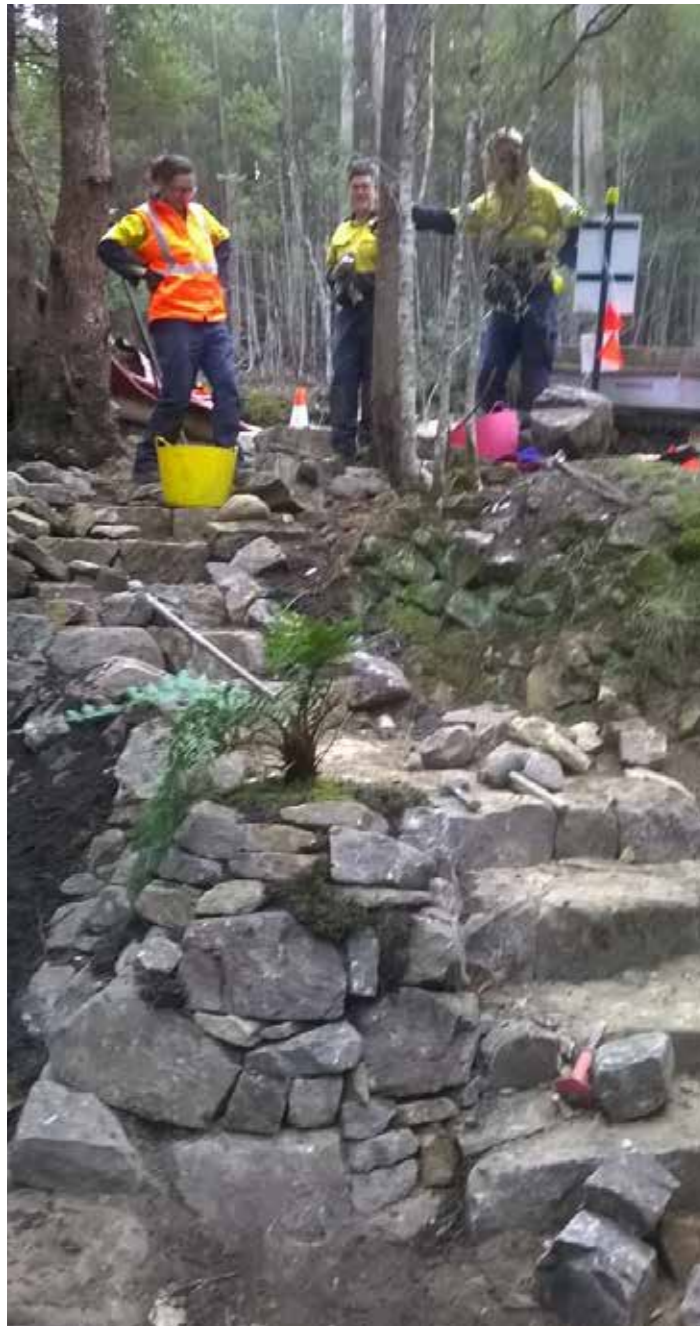
Photo: New steps above Old Hotel site leading to the Pinnacle track
