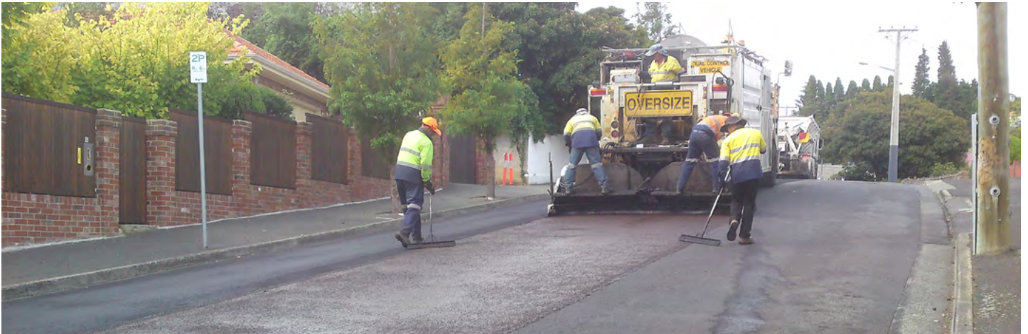
A road crew undertake the resealing process in Lenah Valley, Hobart. Image: The City of Hobart
